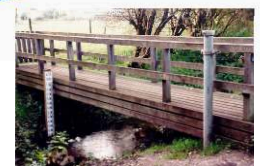
water level measurement with pressure sensor
